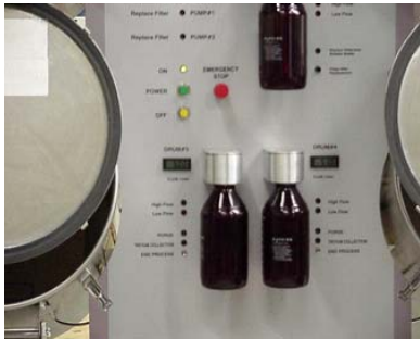
Close up of bubbler and controls
