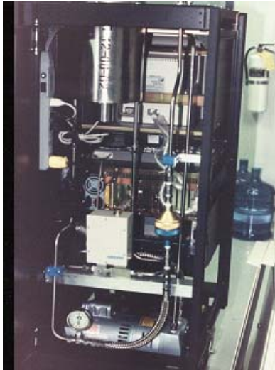
Stack monitor internals
