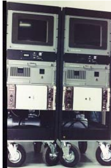
Stack analysis equipment
